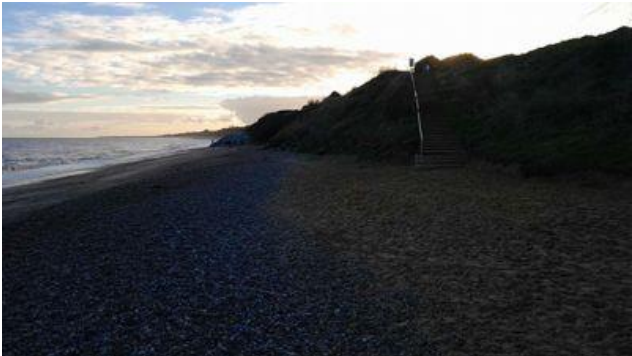
Change in beach level relative to exposed timber groyne opposite Grand Avenue: Moderately lower
